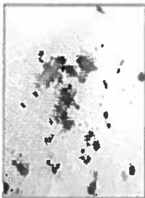
Black or brown stains, usually in crevices
